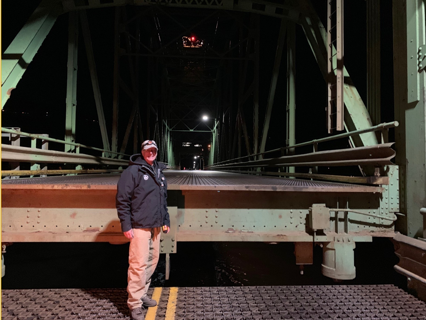
Our “Mann” on the bridge – kudos to Facilities Manager John Mann for so many years of great work.
