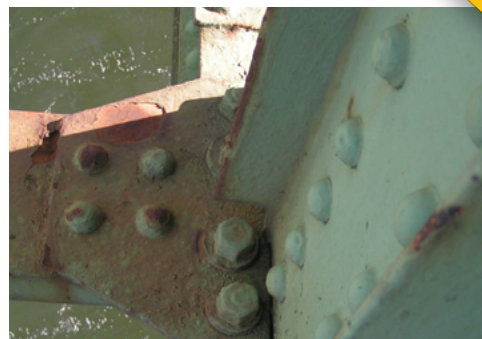
Current steel bridge requires near constant repair
